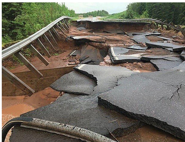
Damage long State Highway 23 near the South Fork of the Nemadji River in Carlton County, Minn., after flash flooding on Sunday. Courtesy of Sgt. Jason Warnygora | Carlton County Sheriff's Office
